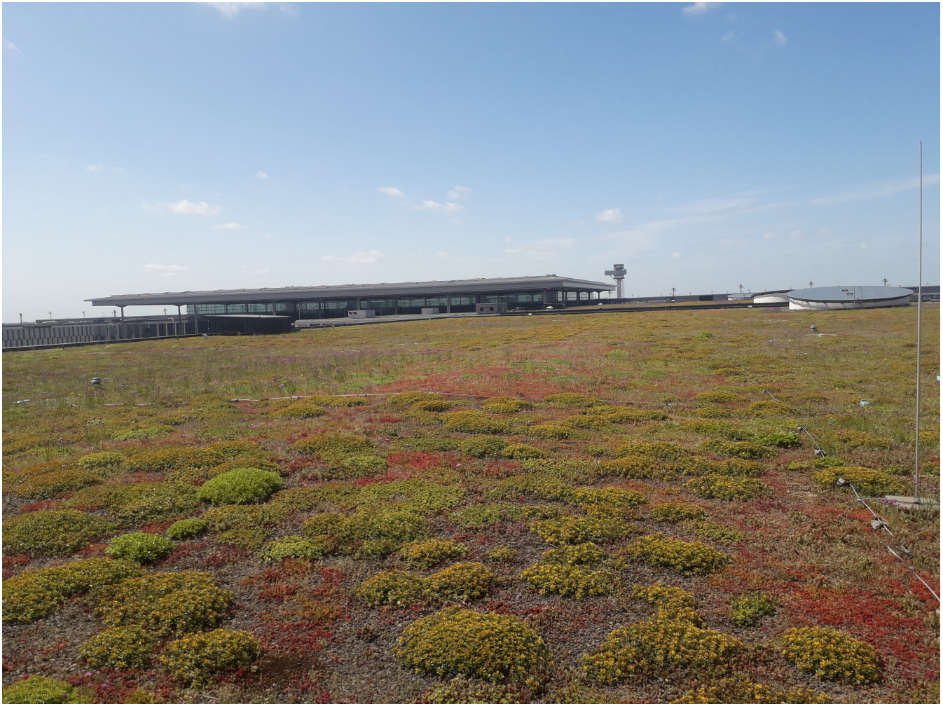
Figure 1. Photograph of the green roof experimental plot located on top of the car park of the Berlin Brandenburg airport (Germany).
