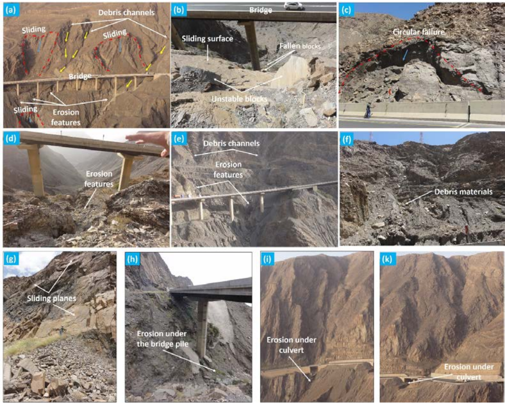
321 322 Fig. 6. Field photographs showing different types of landslides and erosional features along the 323 road section of the study area. a) sliding and erosional features due to running water along 324 gullies, b) Sliding blocks along sliding plane (there are big blocks close to the bridge pile), c) 325 circular failure very close to the bride, d) deep scou re features between bridge piles due to 326 running water, e) debris channels along them erosional features and big boulders appear, f) 327 debris materials of different sizes range from sand size up to big boulders 0.5 m in diameter, g) 328 large planar sliding h) deep erosion and remove the materials surround one bridge pile, i & k) 329 running water remove materials under the culvert make them under risk.
